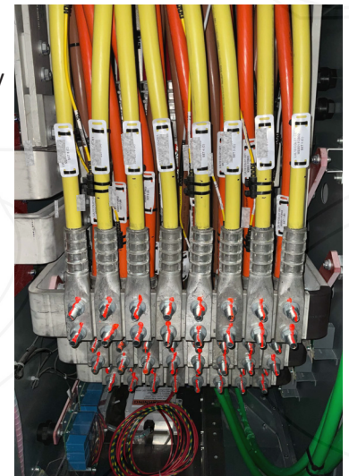
Bellevilles installed on bolted terminals
